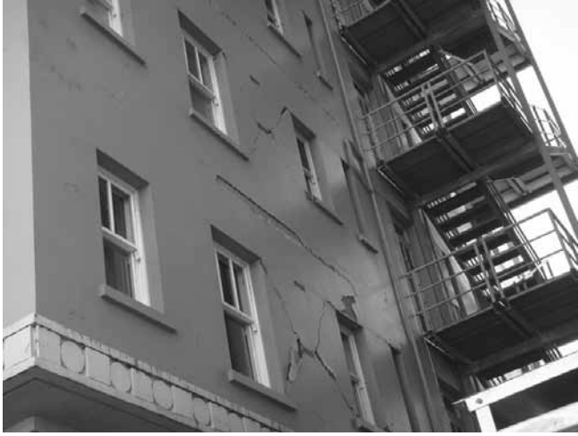
Figure 1. In-plane diagonal tension failure of a URM building caused by the 2010 Darfield Earthquake
