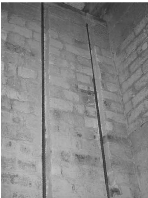
Figure 17. NSM steel reinforcing bars
