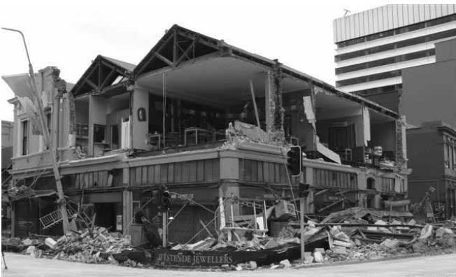
Figure 2. URM building with collapsed walls due to out-of-plane acceleration in the 2010 Darfield Earthquake
