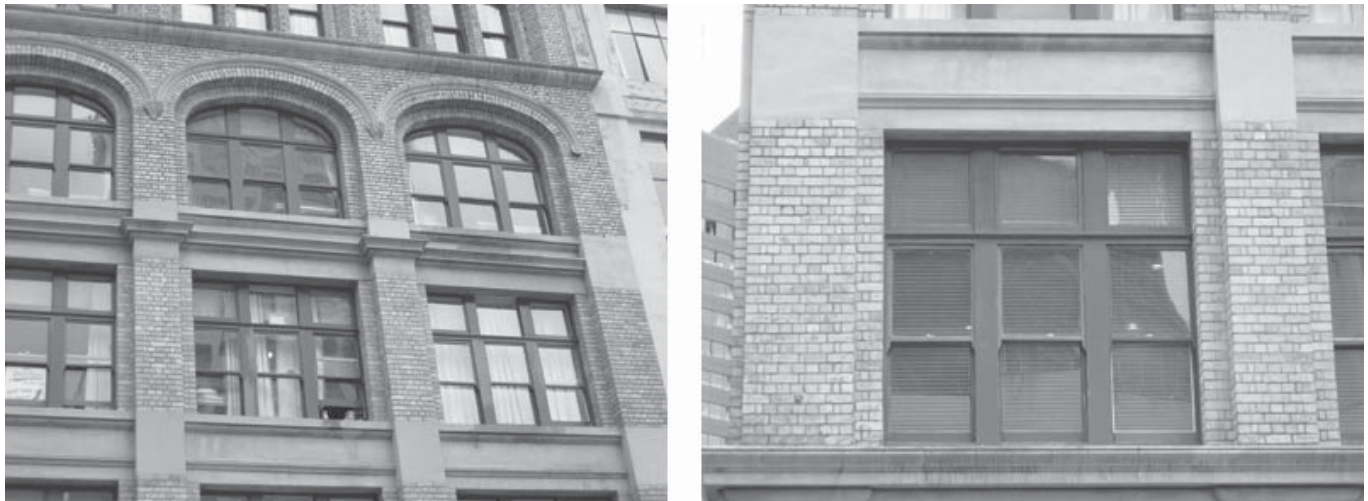
Figure 9. Details of openings. Things to take note of here are the bond pattern and technique used for laying bricks, colouring, striking of mortar, changes in surface, recesses and depressions, and proportions of windows and other components
