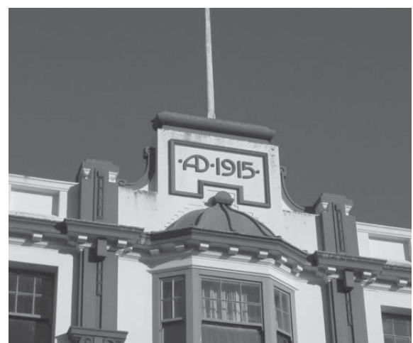
Figure 7. A parapet that is integral with the design of the rest of the facade and which contributes historic information.
