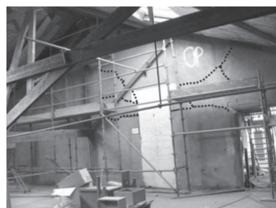
Figure 19. NSM repair – final crack pattern
