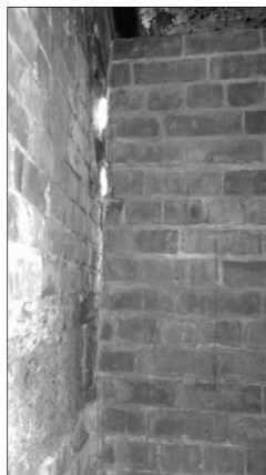
(b) Cracking of the top gable corners (internal view)
