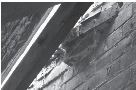
(c) Roof anchor pull-out
