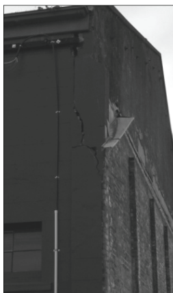
(a) Cracking of the top gable corners
