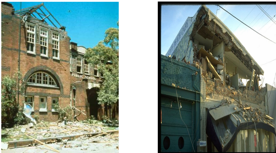
Figure 4 Damage to unreinforced masonry buildings in the 1989 Newcastle earthquake (Australia) (left) and the 1994 Northridge Earthquake (USA) (right)
