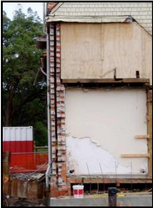
Figure 6 New Zealand multi-leaved wall with change in wall thickness at floor level
