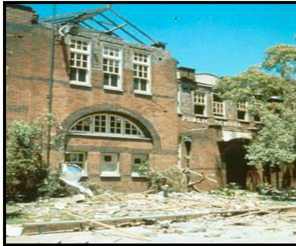
Figure 3: Damage to URM school building in the 1989 Newcastle earthquake (reproduced from [32])
