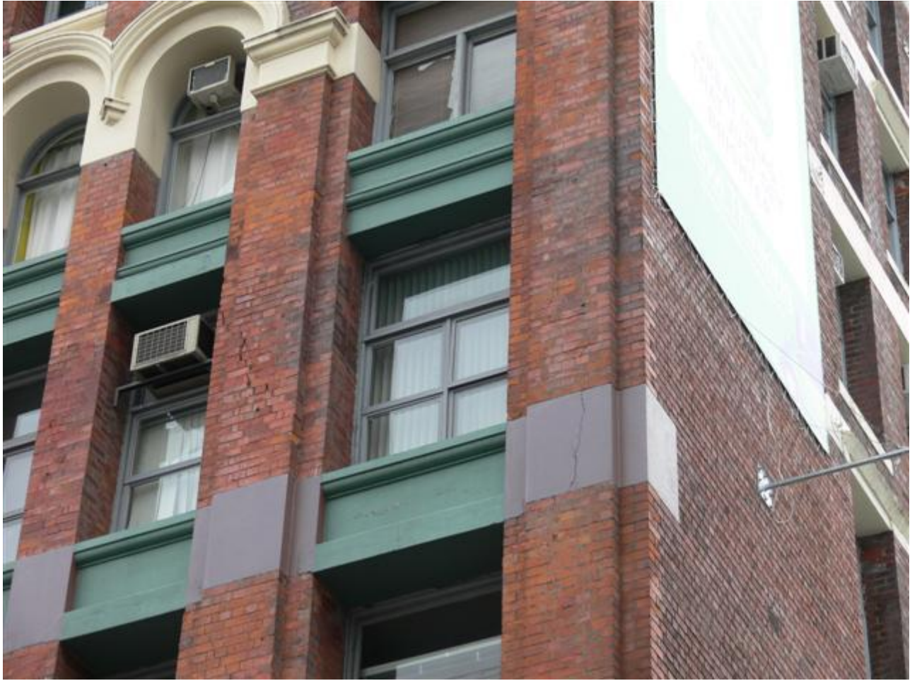
In addition, diagonal cracks at the top of the rear walls suggested that the building had been subjected to torsional deformations during the earthquake.
